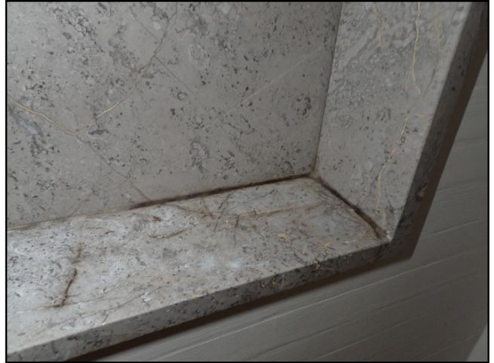
Caulking deteriorated / discoloured
